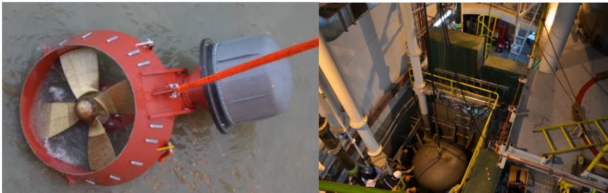
Azipod CZ thruster with dome during UW mounting and the corresponding slightly larger dome in the vessel thruster room
