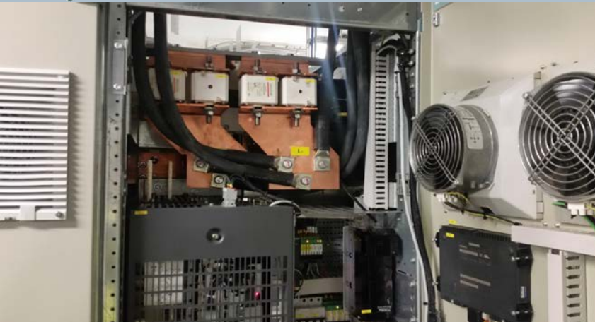
Cables connected below fuses, motor module for FiFi pump disconnected
